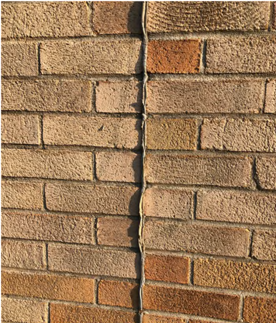
Photo 2: Close-up of the caulk present at the northern exterior wall.
