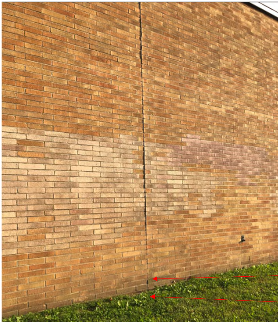
Photo 1: View of the caulk and soil sample locations at the northern exterior wall.
